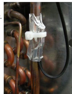
Thermistor attached to the refrigerant line.
