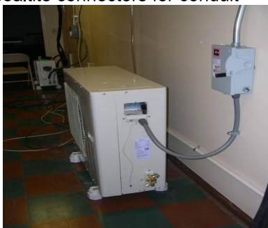
Local Disconnect and Whip Connected
